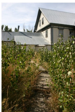
Overgrowth that needs clearing
